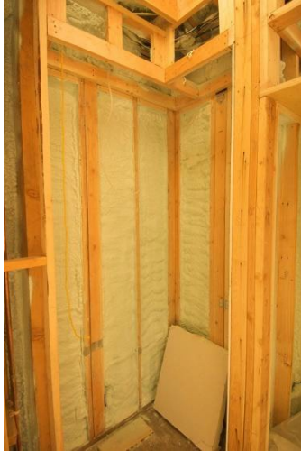
Figure 14.8: Insulation is used to limit the conduction of heat from the inside to the outside (in winters) and from the outside to the inside (in summers). (credit: Giles Douglas)
