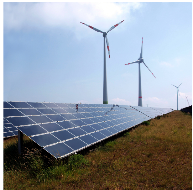
Figure 3: Photograph of Solar Panels and Wind Turbines.
